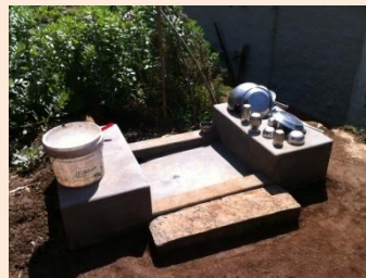
Soak pit washing station
