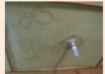
Leaky roof in school computer room
